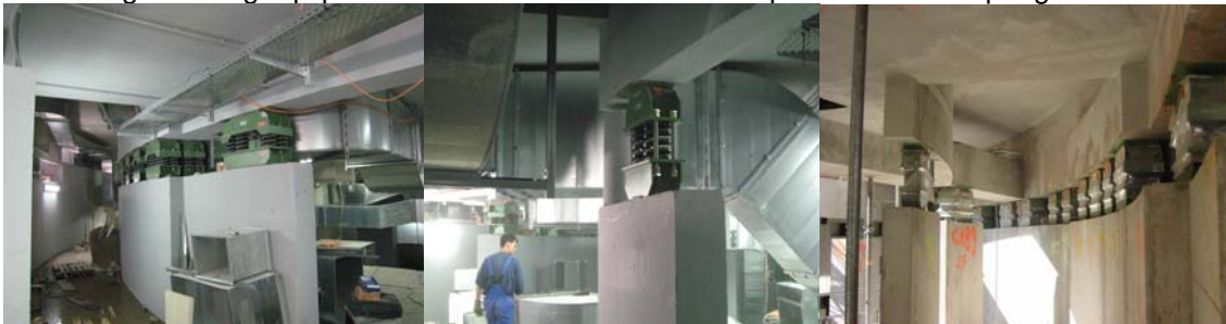
Figure 14.-Views of spring systems under the 20000-ton opera house
