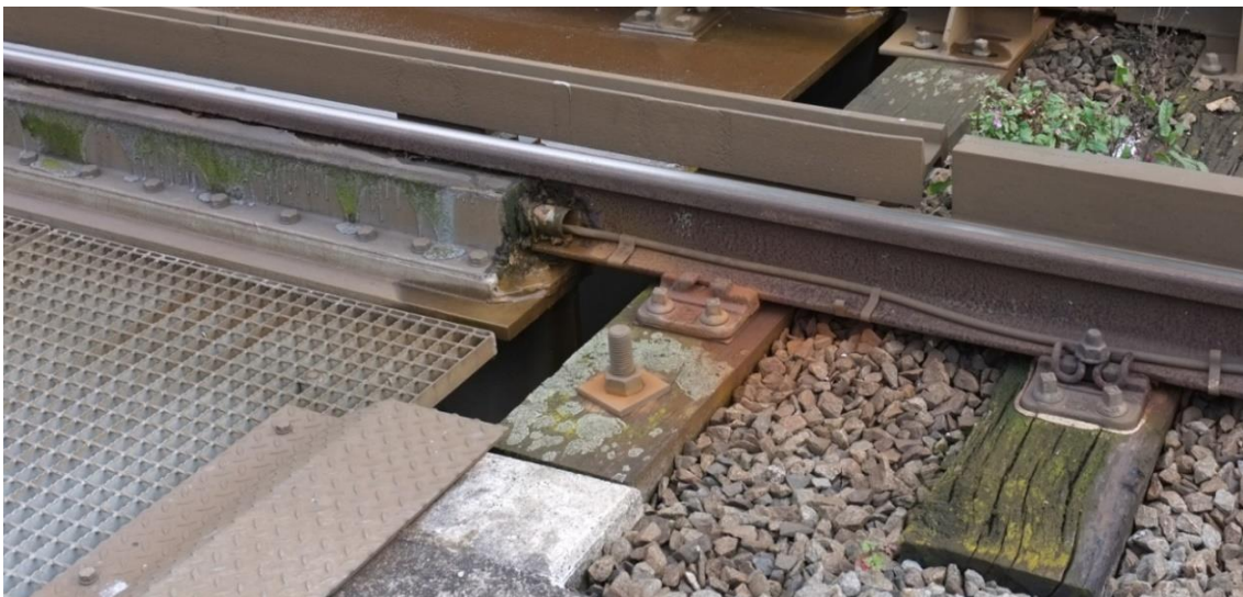
Figure 4 Transition from embedded rail (left) to ballasted track (right) on a steel bridge across the river Roer in Roermond. Photo by Movares.
