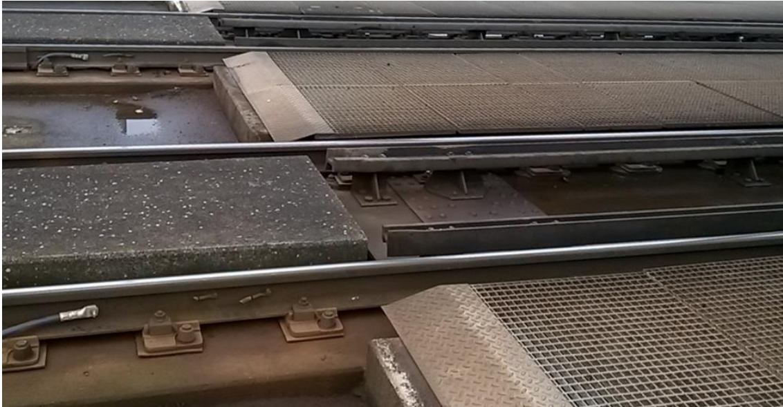
Figure 3 Direct fastening on concrete (left) and steel parts (right) of the large bridge across the river IJssel in Deventer. Photo by Movares.
