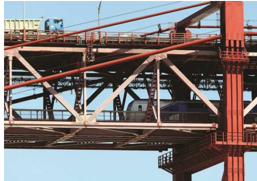
Figure 1 –View of the rail and road platforms of the 25 de Abril Bridge
