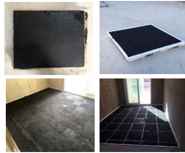
(b) MSK2 Installation
