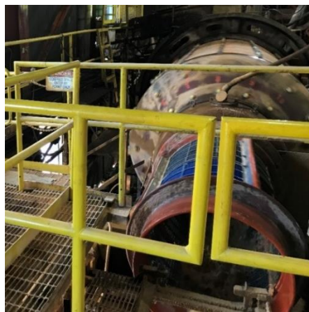
Figure 9: Rod mill located inside the processing building
