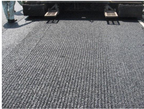
Photograph 3 - Example of road-laying using a longitudinal groove rough surface hybrid pavement -dedicated AF
