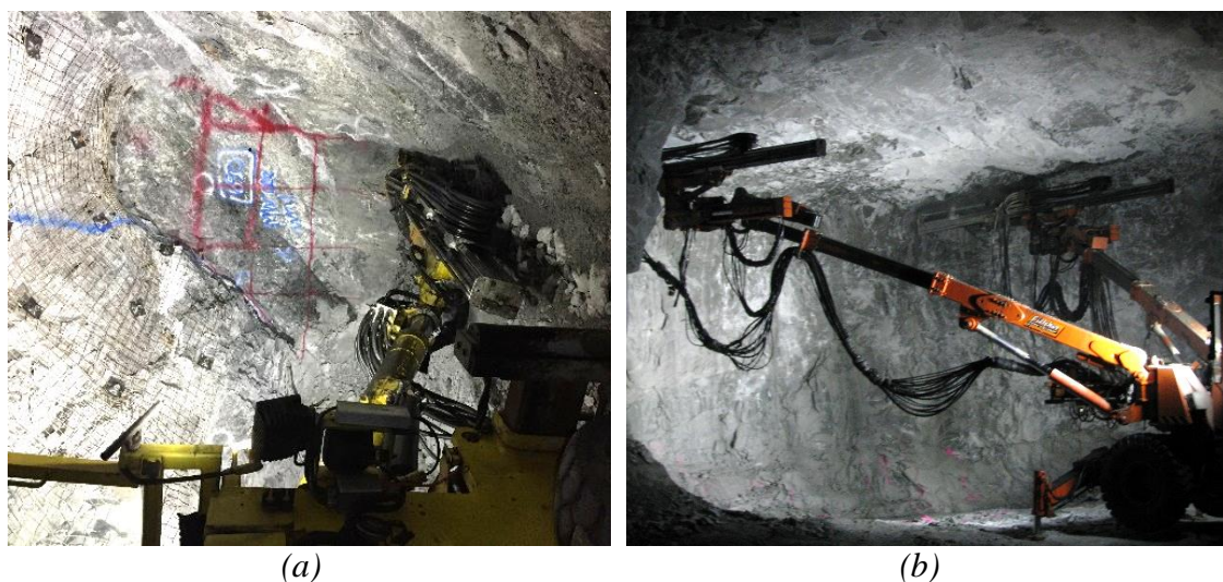
Figure 2. Field test setup used in (a) Mine A (single-boom), and (b) Mine B (dual-boom).
