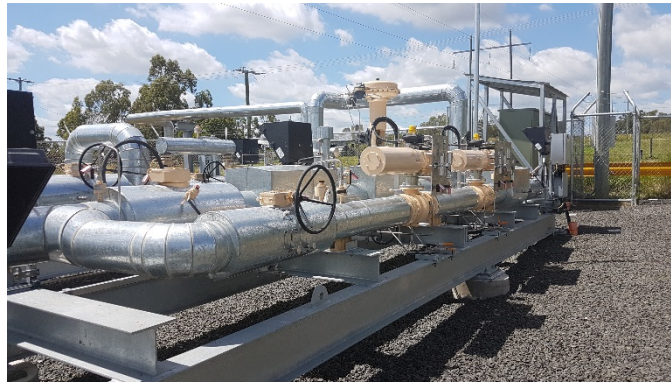
Figure 7: Acoustically insulated PRS pipework
