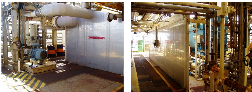
Figure 2: Incorrect noise control applied to pipework and water injection pump
