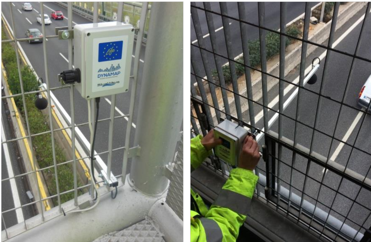
Figure 6. View of a HCCS installed on top of a portal.
