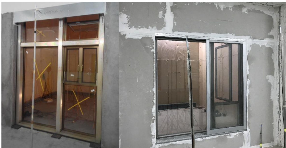
Figure 1 Test windows installed with brick Walls (left) and carcass made of gypsum boards with infills (right)
