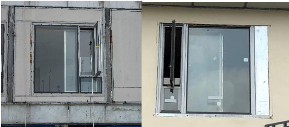
Figure 2 Test windows installed at testing facades with concrete sandwich panel (left) and metal sandwich panel (right)
