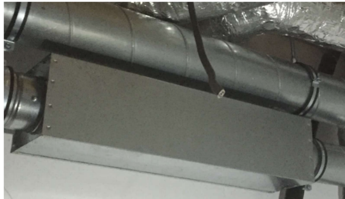
Figure 3 Galvanise steel silencer installed in residential ventilation system
