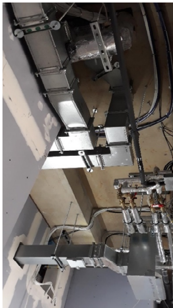
Figure1 Typical galvanised steel duct installation for the residential whole house ventilation
