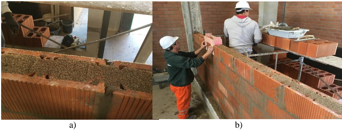
Figure 2: a) Construction of the test specimen on portico system; b) Filling of the block cavities with vermiculite.
