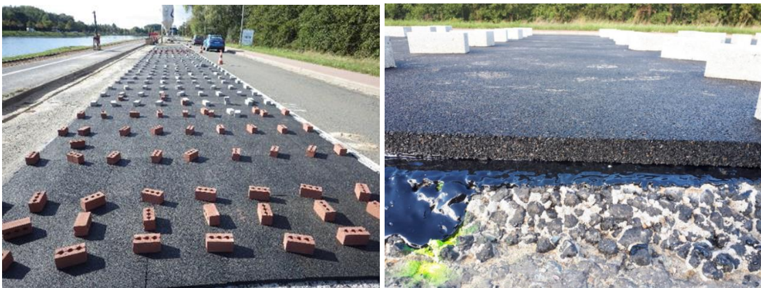
Figure 7 Curing PERS test track with bricks on the corners to avoid curling up of the slabs
