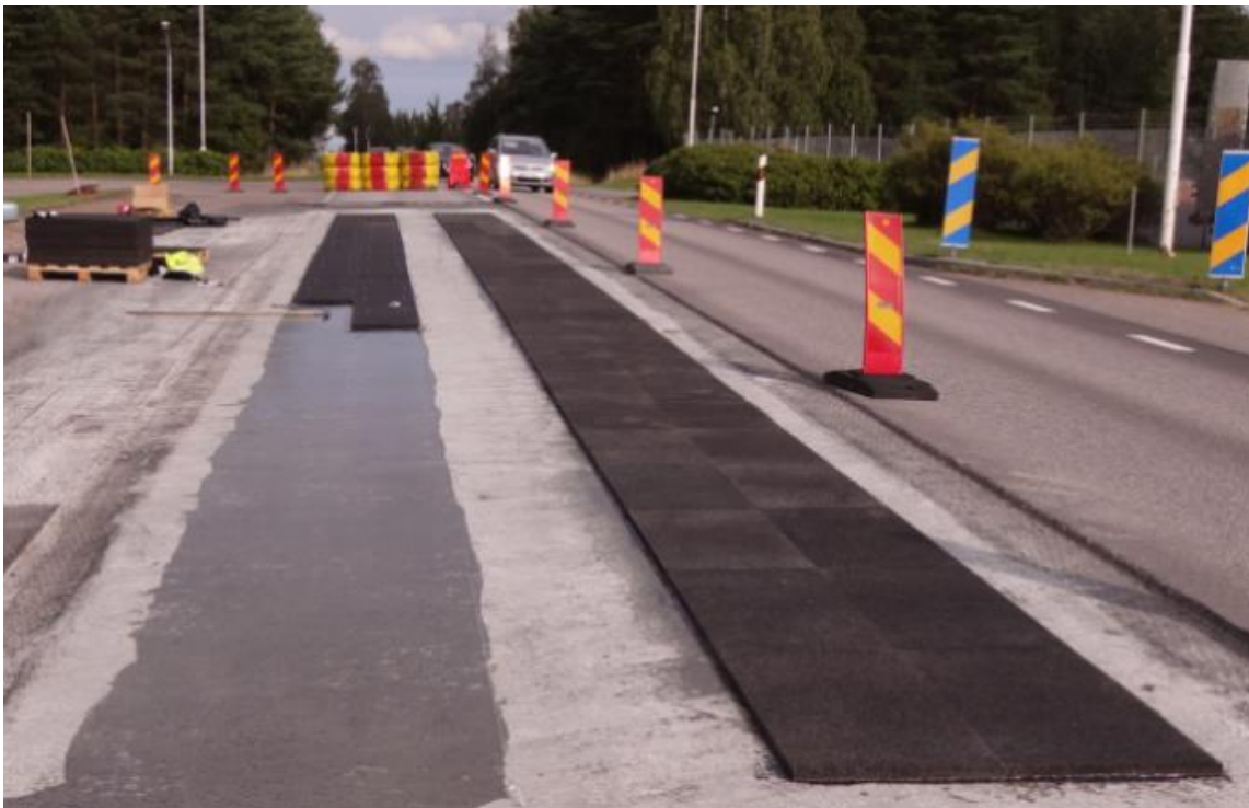
Figure 1 The PERS track in Sjögestad (two strips in wheel tracks) under construction (photo: courtesy of Ulf Sandberg, VTI)
