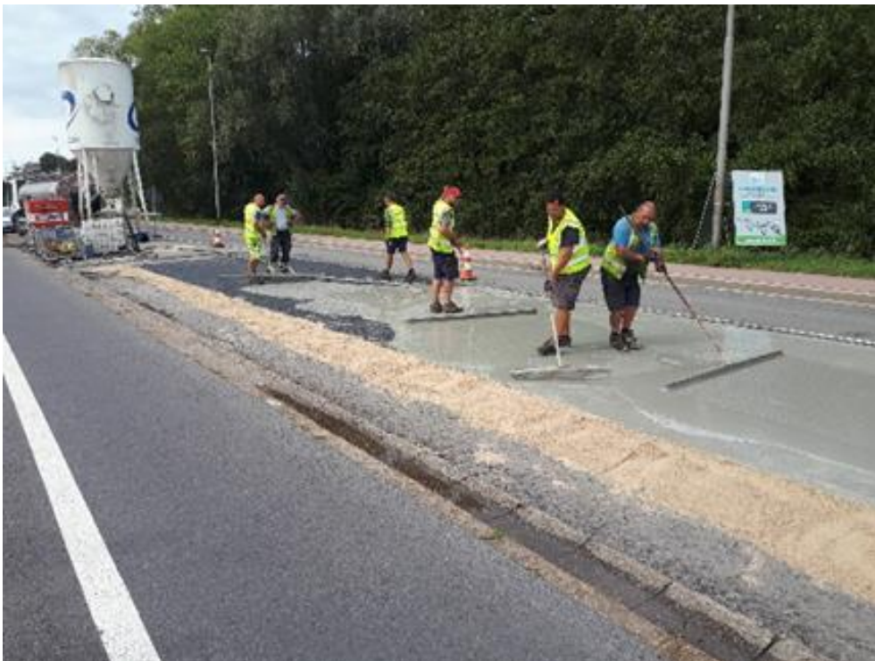
Figure 5 Filling of the voids of the porous asphalt layer with cement slurry
