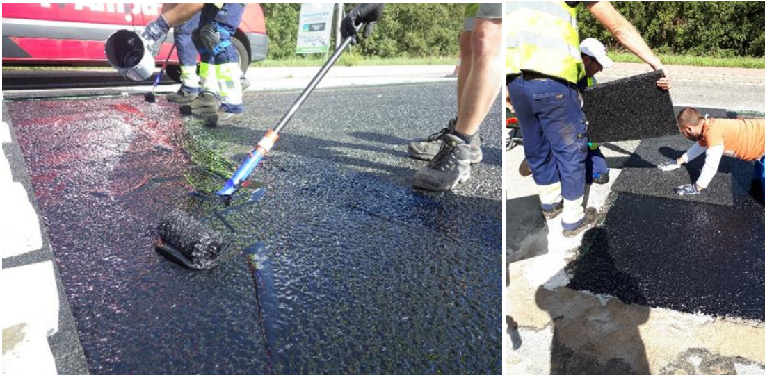
Figure 6 Application of the glue (left hand side) and manually laying of the slabs
