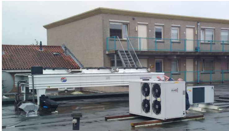
Figure 3: installation of condensing unit of the shop roof and at proximity of the neighborhood – proximity with living place created troubles and action was required to minimize noise from the units.
