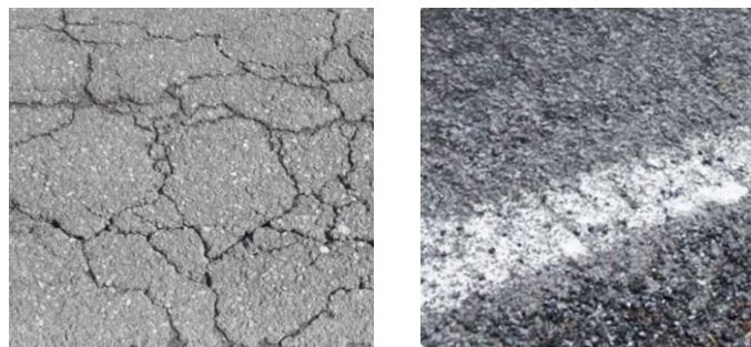
Figure 1. Example of pavement with alligator cracking (left) and ravelling (right)
