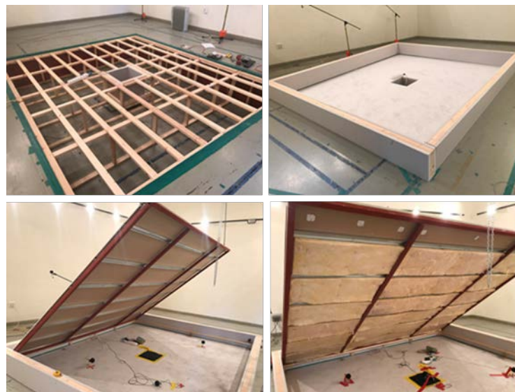
Figure 2. Installation of mock-up ceiling system and glass wool in the reverberation chamber
