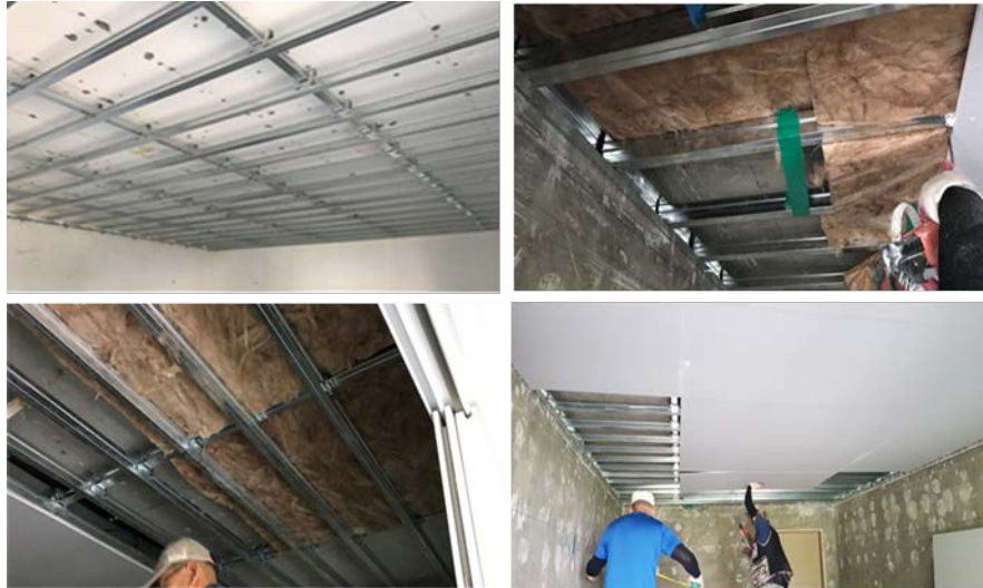
Figure 4. Installation of mock-up ceiling system and glass wool in the test building
