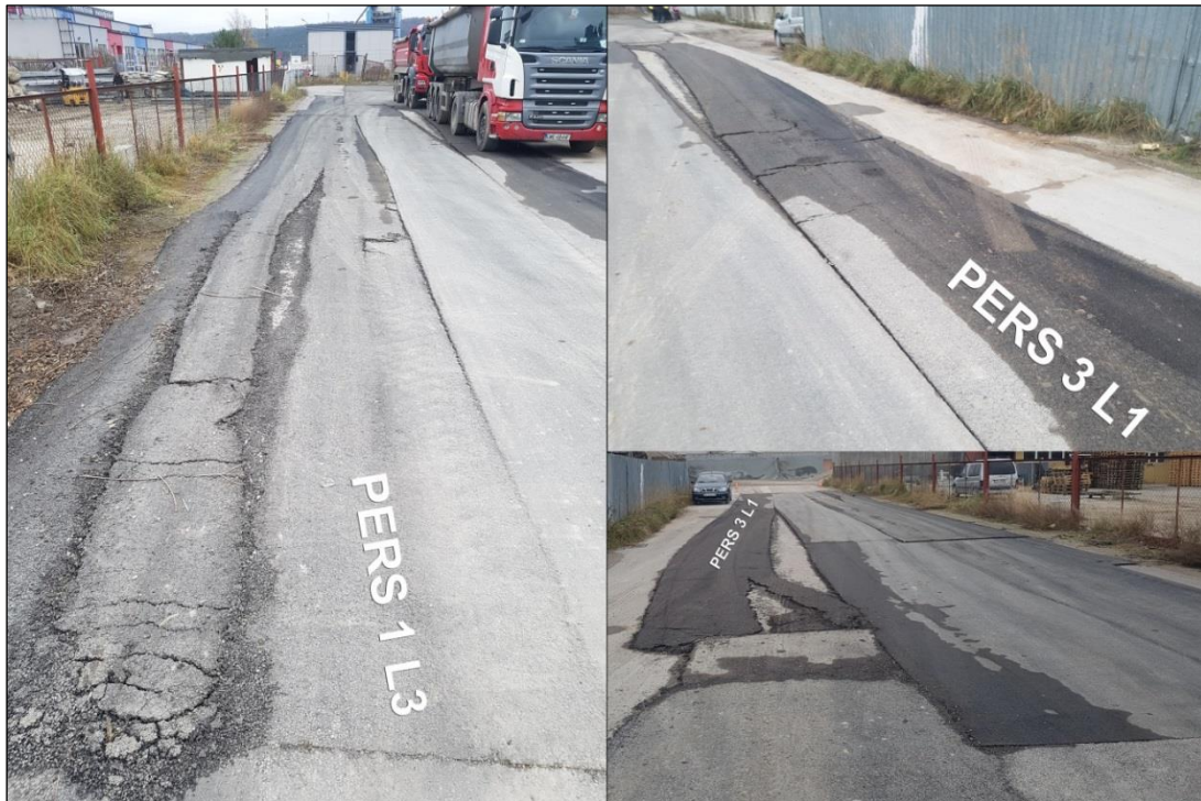
Fig. 4. Technical condition and damages of PERS test sections
