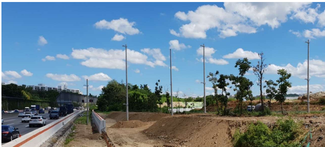
Fig.05 Picture of noise meters installation
