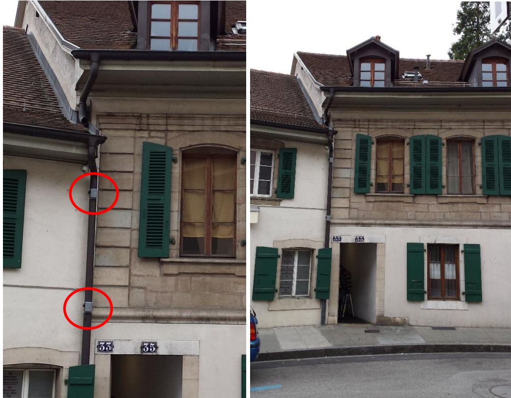
Figure 6: View of ANS installation on the buildings' facades
